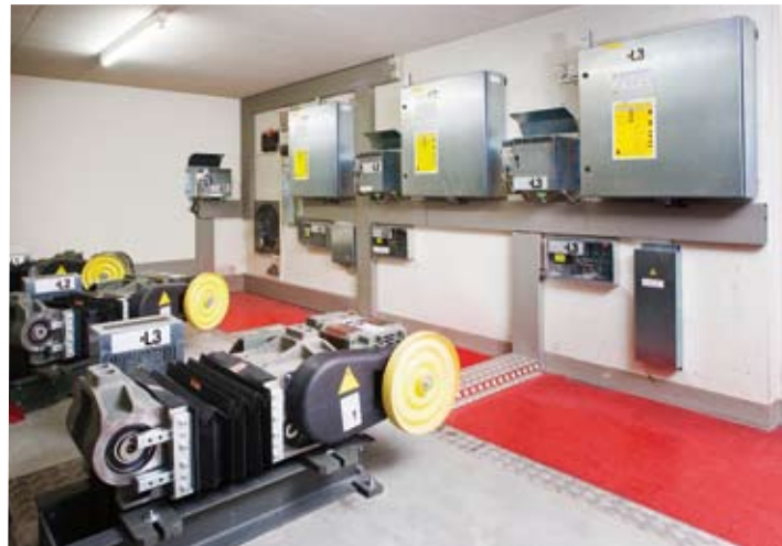
Triplex commercial installation powered by DR SGB 142 linked with a CO MX control
