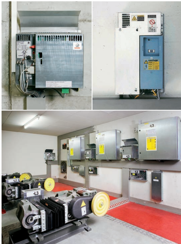
Triplex commercial installation. DR VAB frequency converter linked with a CO MX controller. Powered by DR SGB 142 machine.
